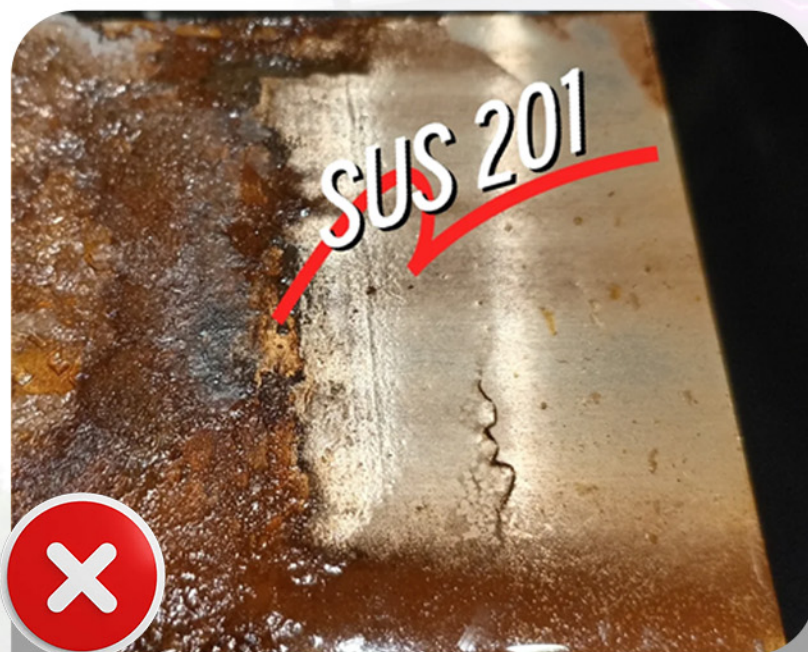
201 STAINLESS STEEL 2 YEARS OF RUST AND CORROSION.
